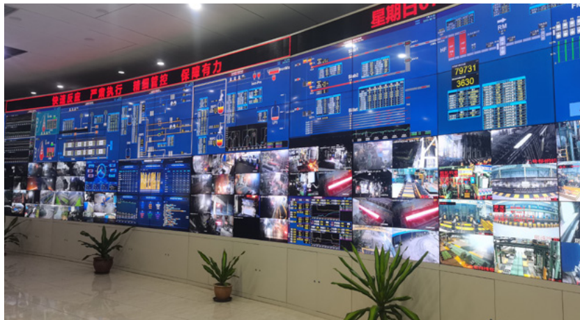
Energy Management System Monitoring Centre
